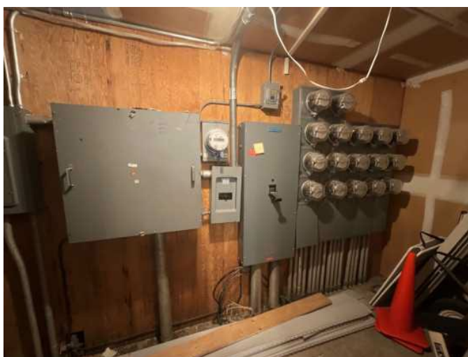
17 - MAIN ELECTRICAL ROOM
