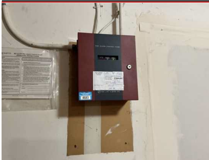
19 - FIRE ALARM PANEL
