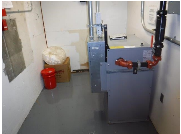
4. Machine room is clean and organized.
